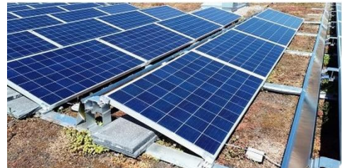
Abb.3: Solarpanels wandeln Licht in Strom um.
